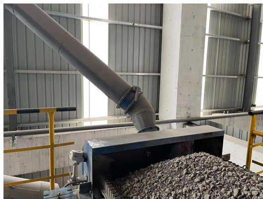
破碎粉尘进料点粉尘废气密闭集气罩
